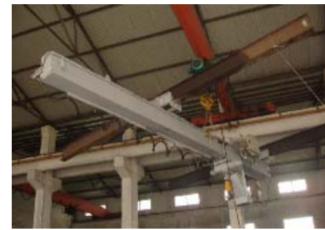
EXTEND BEAM ENGINE ROOM CRANE (ODES)
